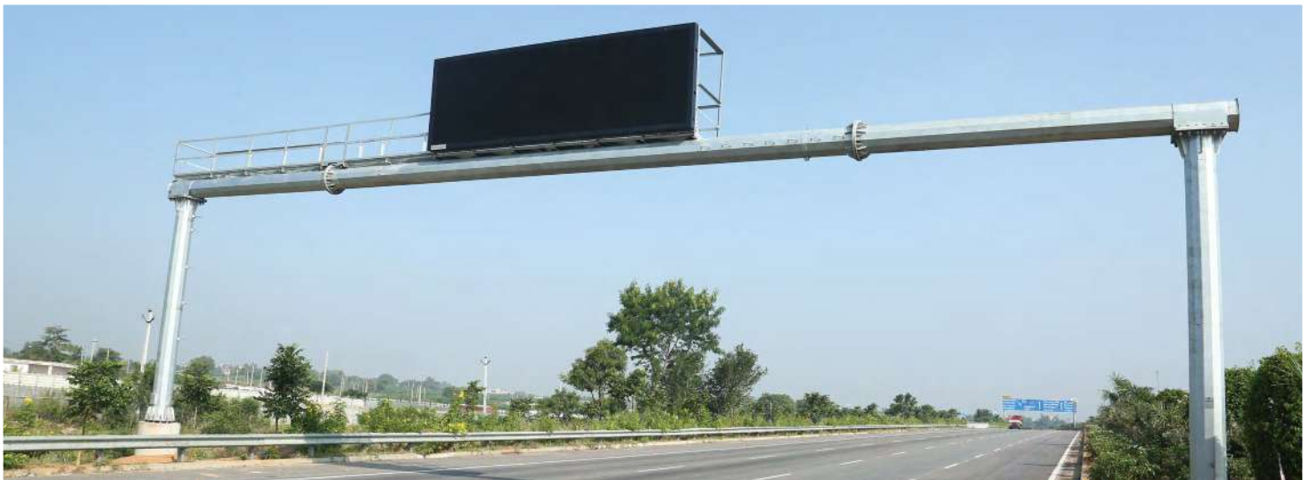
(TOP LEFT) F-TYPE CANTILEVER INSTALLED AT HYDERABAD OUTER RING ROAD; (TOP RIGHT) TRAFFIC SIGNAL STRUCTURE INSTALLED IN PUNE & (BOTTOM) GANTRY INSTALLED AT HYDERABAD OUTER RING ROAD
