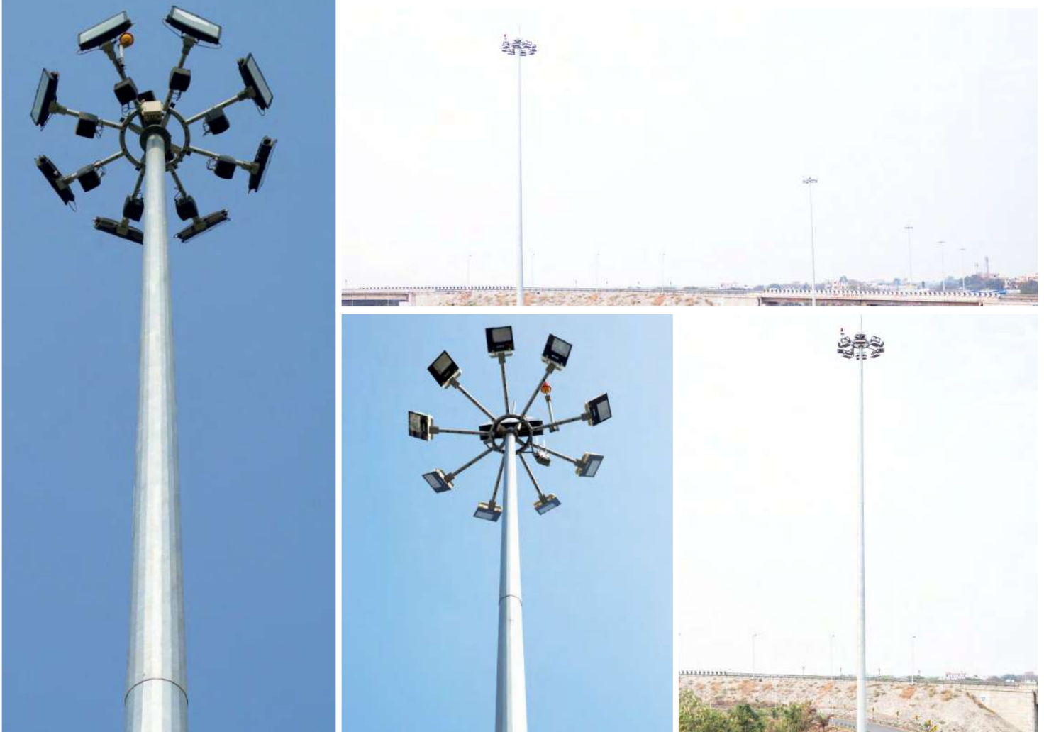
HIGH MASTS INSTALLED AT INDAPUR, MAHARASHTRA AND HYDERABAD OUTER RING ROAD
