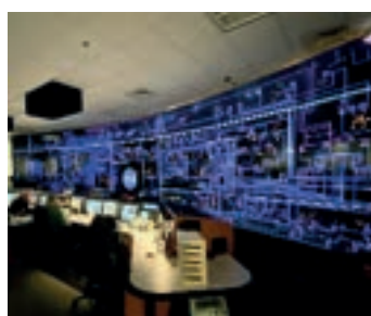
Control Room Setup
